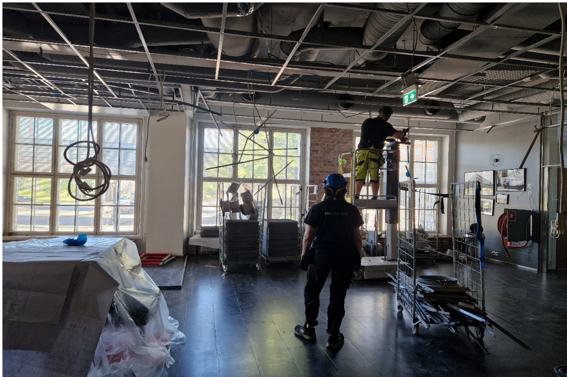
Figure 19. Deconstruction worker cutting and taking down T-lists was interviewed on their intact deconstruction and subsequent reusability. The metallic false ceiling grids that laid on the T-lists were taken down earlier.
